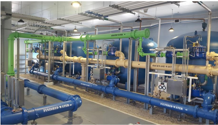
The new filtration plant at Memorial Beach.
