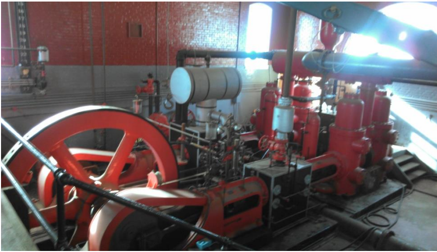
Steam Driven Pump - Memorial Beach Station 1 circa 1800s
